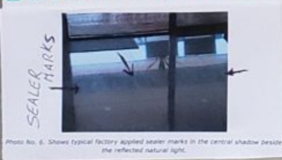
Photo No. 6. Shows typical factory applied sealer marks in the central shadow beside the reflected natural light.
